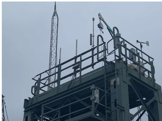
Example of guardrails around a walking / working surface higher than 4' above the next level.
